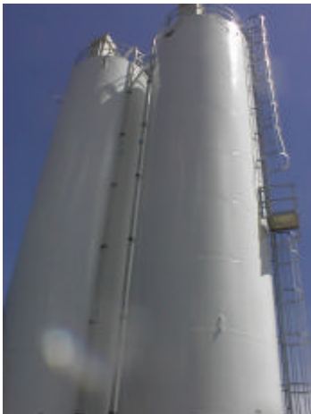
Raw Material Storage Silos
